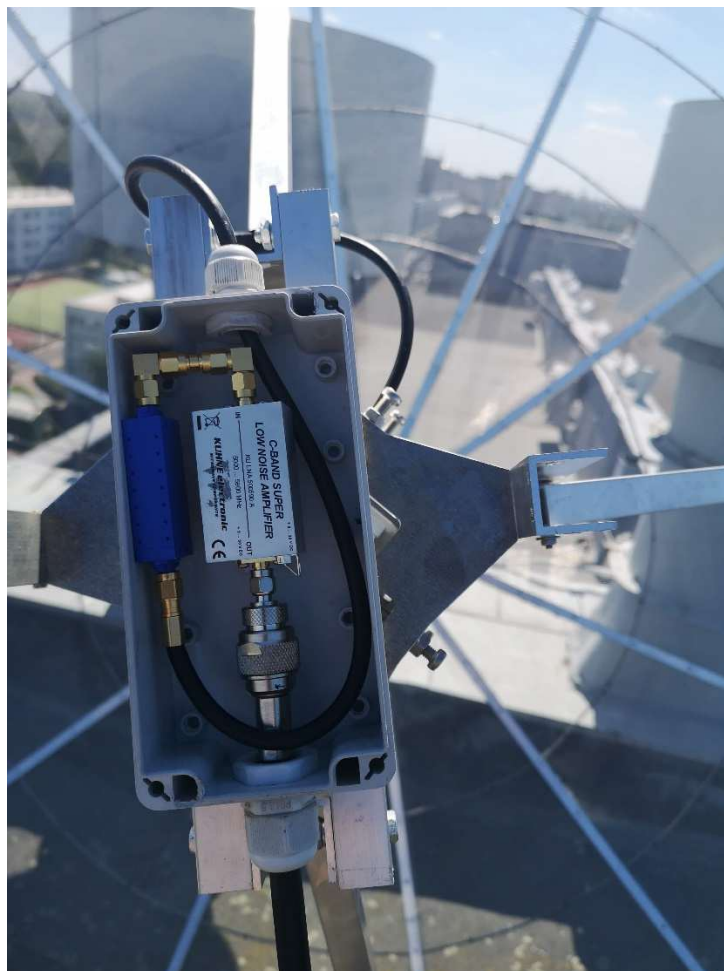
Fig. 1.6 Antenna pre-amplifier in a water-proof housing
